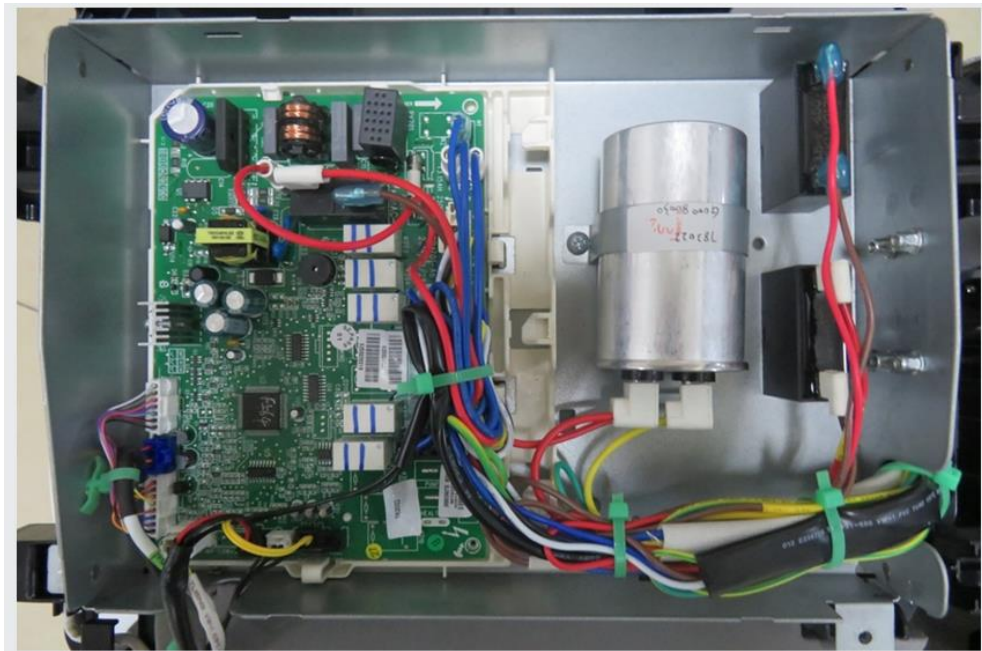
Main PCB M701F1NJ (Electrical box view)
